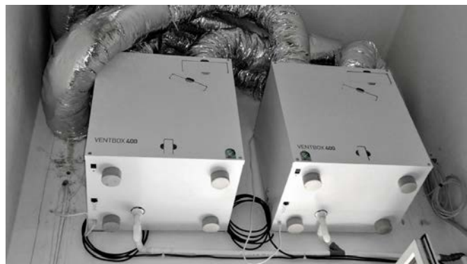
Two ventilation units with heat recovery (VENTBOX 400)
