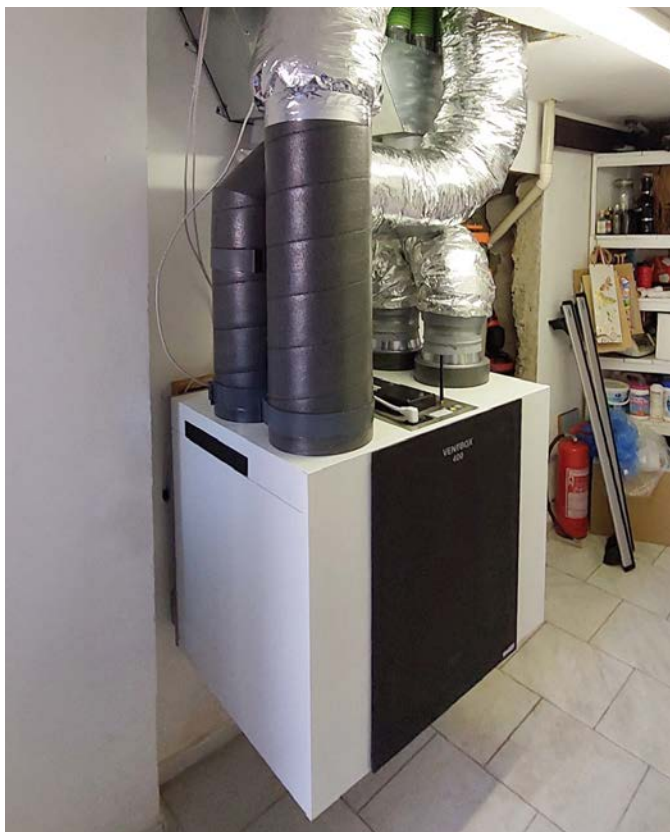
Installed VENTBOX 400 unit in the utility room
